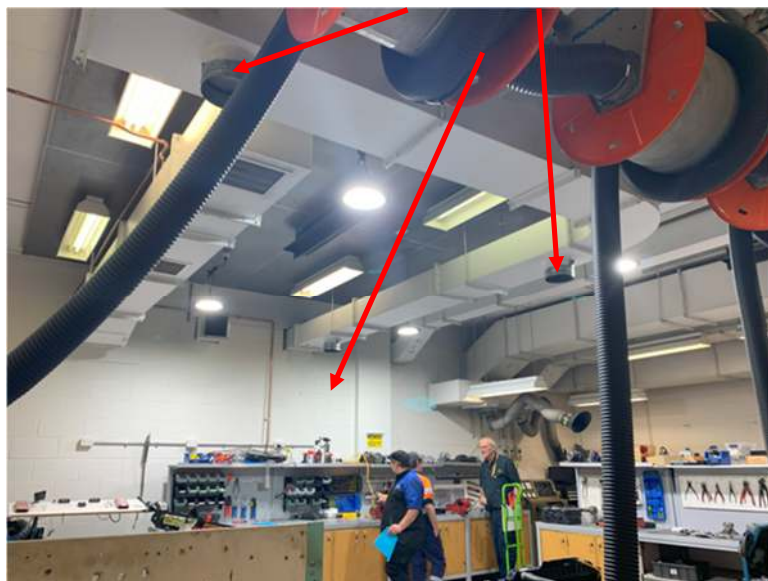
Figure 5 location of unsealed ducts The majority of stand mounted engines in the AG-01 workshop area are only operated for a short period of time.
